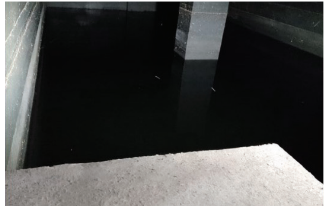
Rainwater tank at Basement 3
