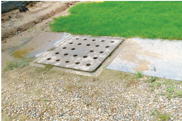
Storm water connection outside building premises
