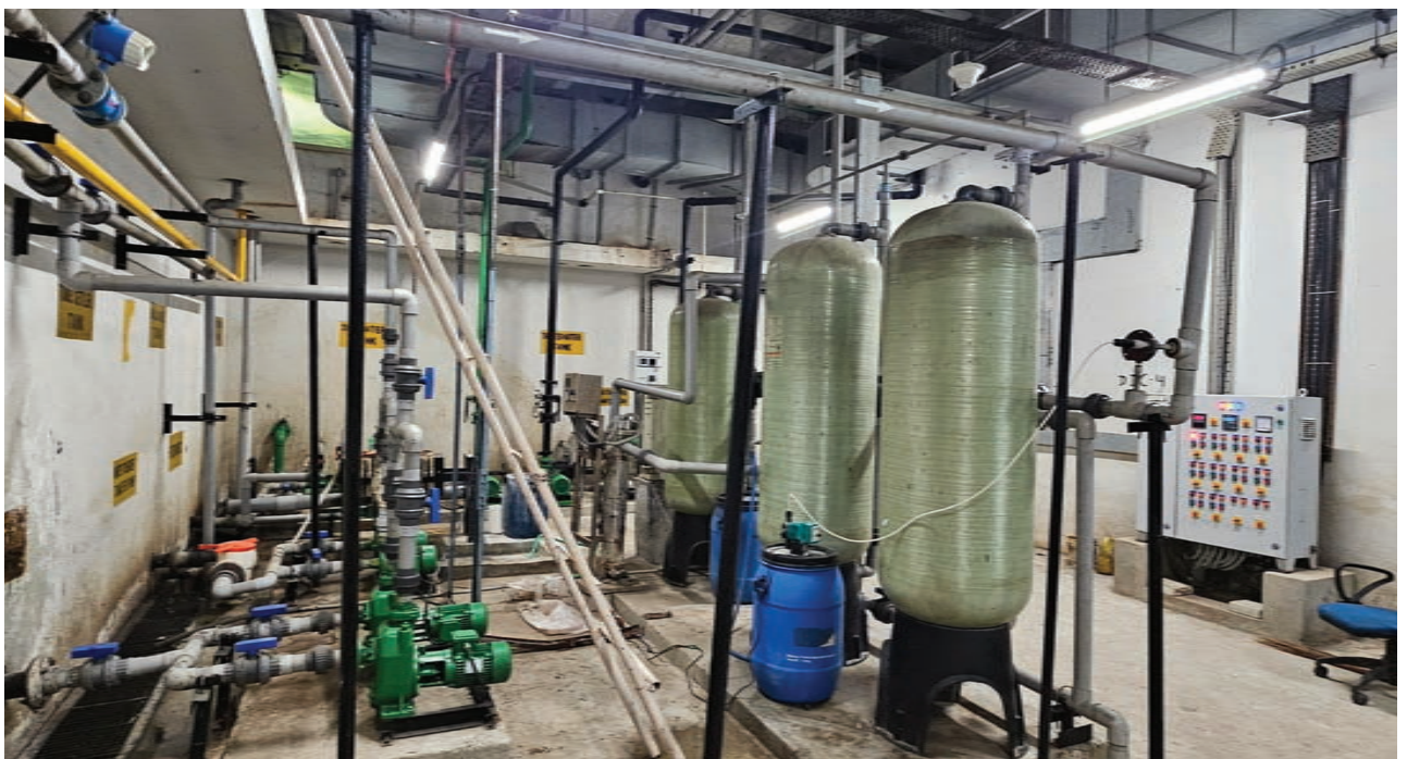
Sewage Treatment Plant (STP)
