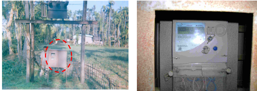
Fig 3.4: Energy meter installed at transformer under SPSS system
