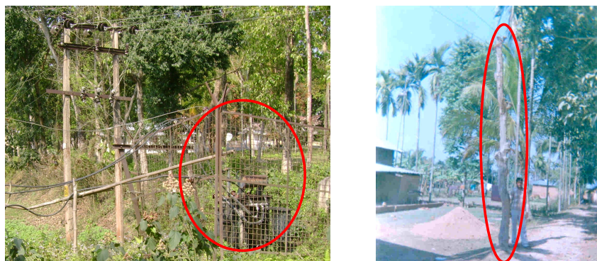
Fig 3.6: A view of the distribution network
