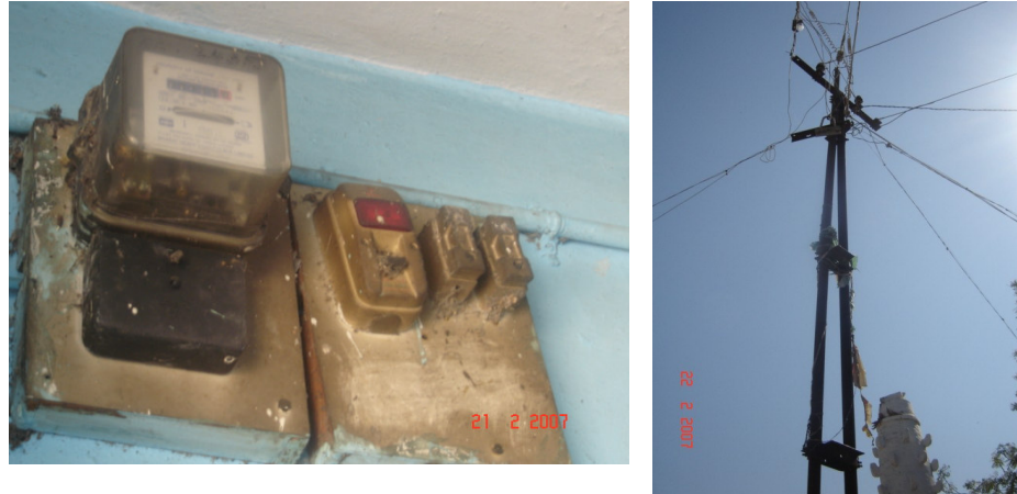
Figure 4.2: Condition of existing power sector infrastructure in Gulbarga district
