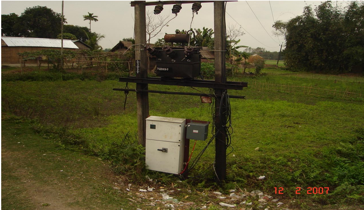
63 KVA Transformer, Village: Tapattary
