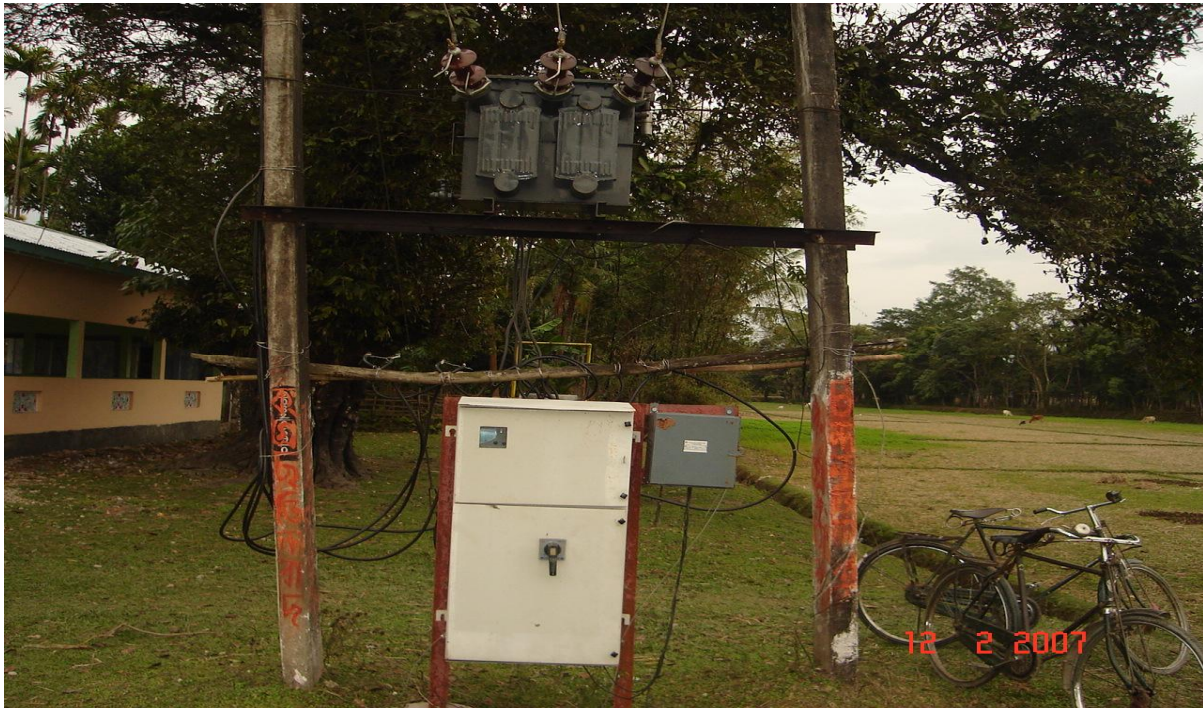
63 KVA Transformer, Village: Haripur
